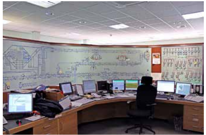
The Metro Control Centre at South Gosforth. Photo Llangollen Signalman
